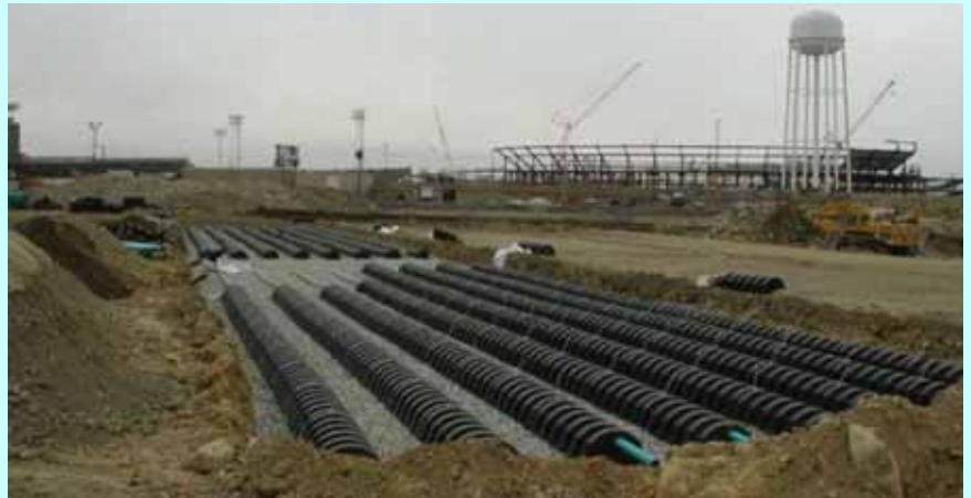
Stormwater disposal chambers installed under parking lots at Gillette Stadium treat excess wastewater and stormwater.
